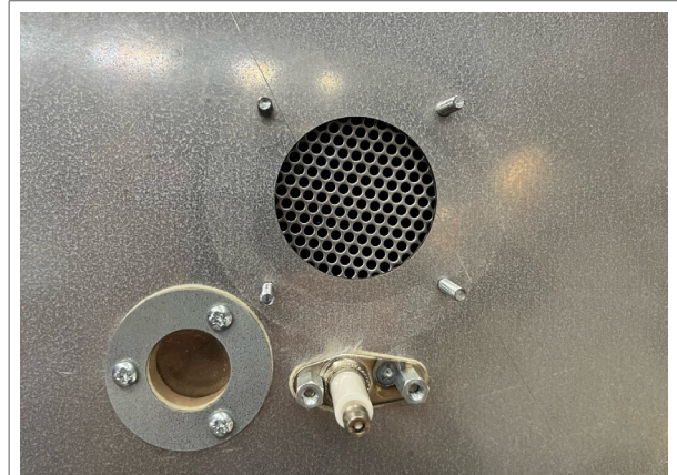
Figure 23 - The grid in front of the burner
