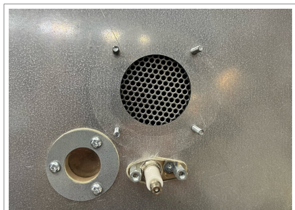
Figure 32 - The grid in front of the burner
